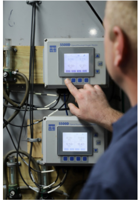
Two of the 5500D monitors installed at the facility
